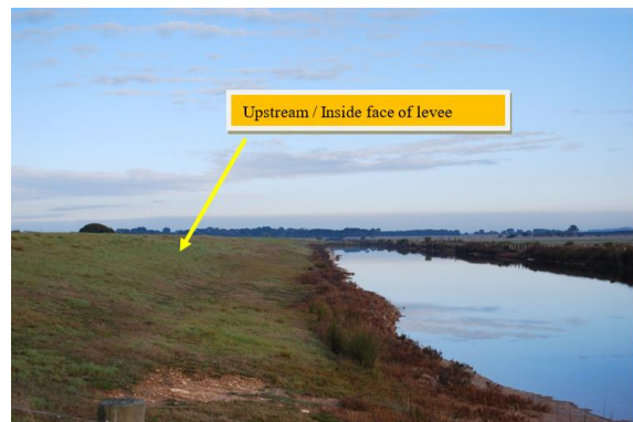
Site Photo of the Plummer Bank Levee showing borrow pit on upstream (river) side
