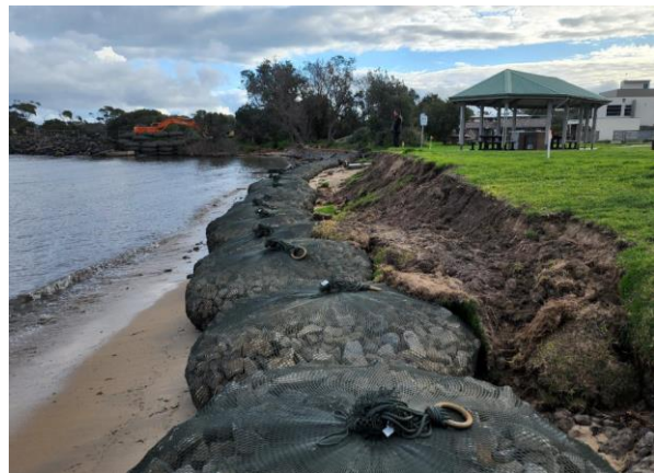
Toe layer of Rock Bags laid out during construction process (source: engage.basscoast.vic.gov.au).
