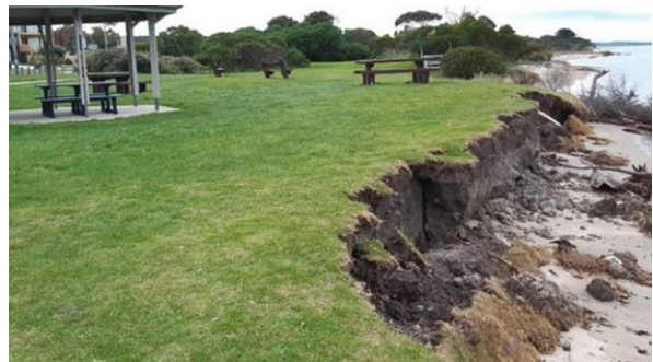
Pymble Ave reserve shoreline erosion before Rock Bags were implemented.
