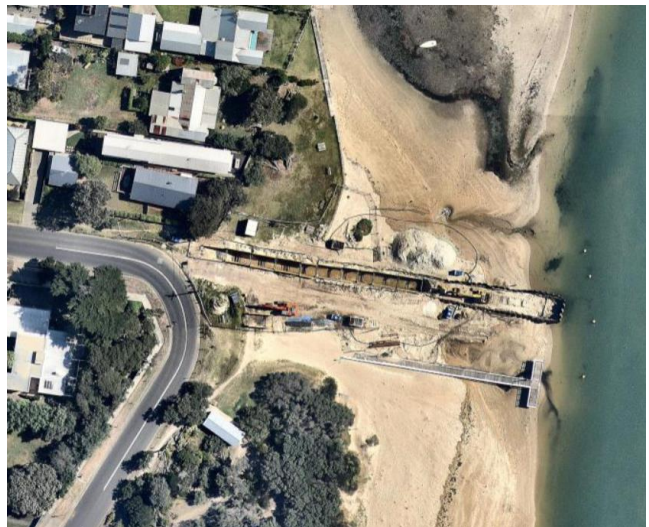
Construction of the outfall opposite the junction of Flinders parade and Ozone Street, Barwon Heads in 2017
