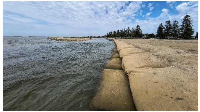
Figure 4 Recently constructed geotextile training wall to redirect flows away from Altona seawall
